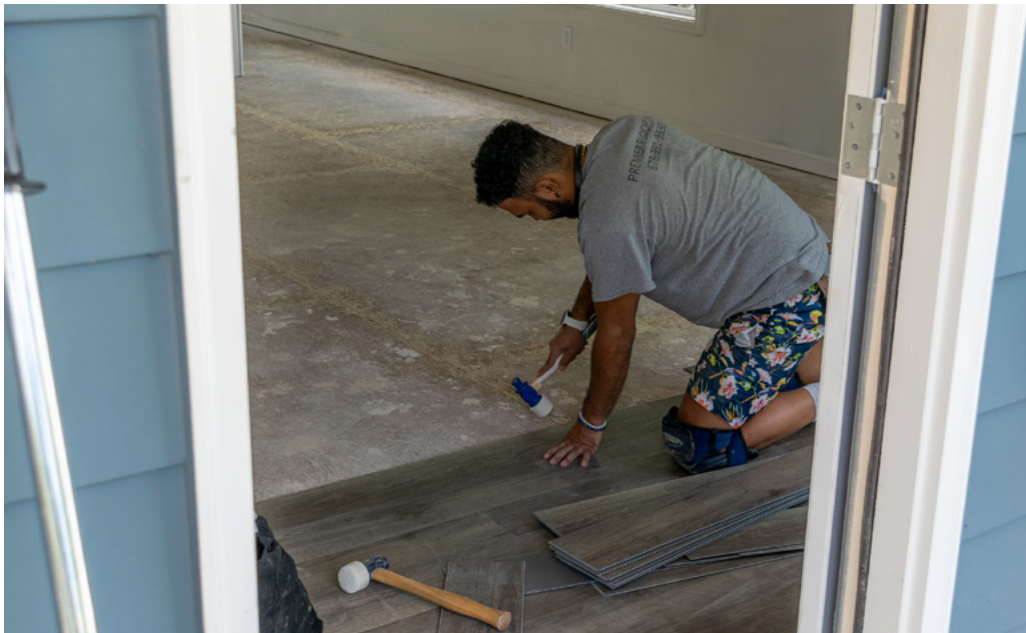
A builder installs flooring on an infill home getting ready to be sold by the Atlanta Land Trust. (Photo: Community Progress)
