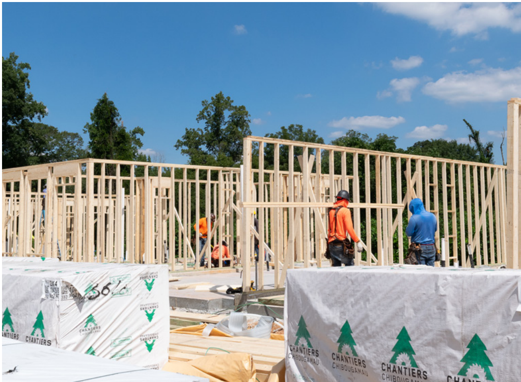
A building crew works on the framing of new affordable homes in Atlanta. (Photo: Community Progress)
